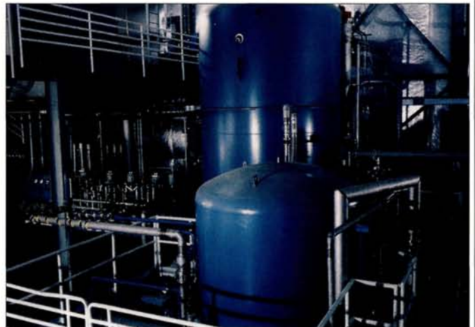
When JLab's central helium liquifier came online in 1993, it doubled the world's cooling capacity at 2K to 4.8kW.
